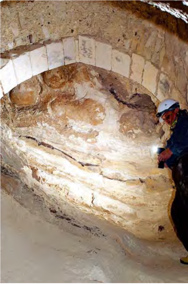
Fig. 9 - Part of the masonry supporting the helical section (photo C. Germani, E. Burri).
