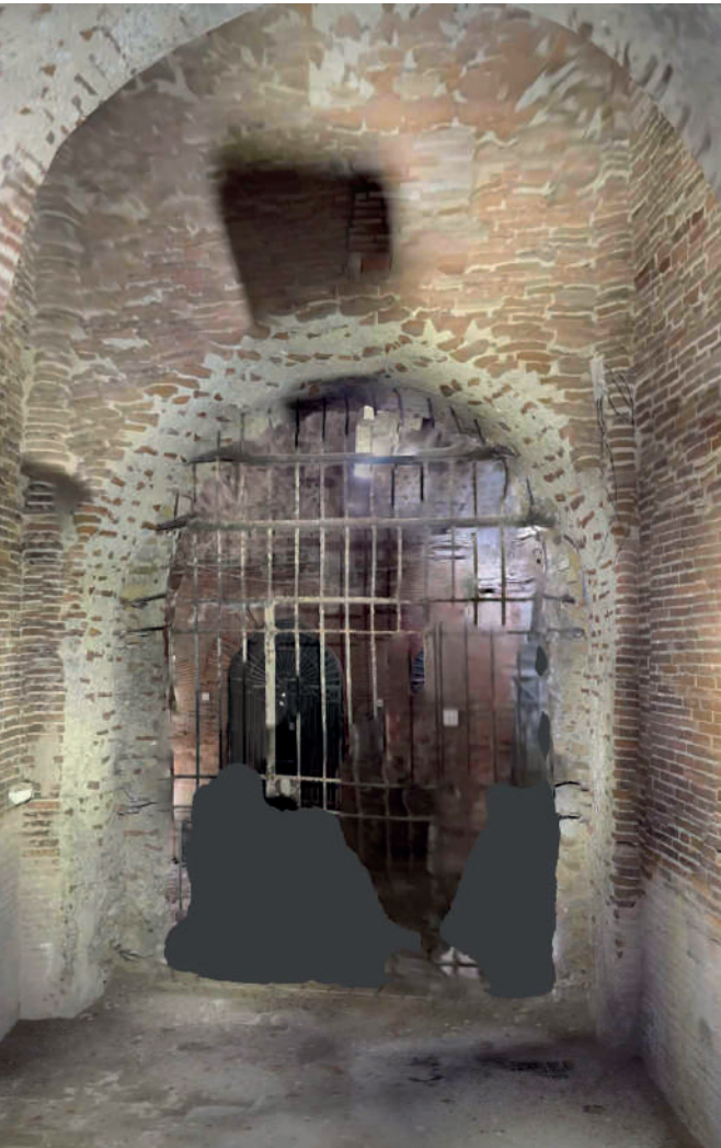
Fig. 5 – Issues in scan results: device shadows (top), iron gates and missing scan areas (bottom).
