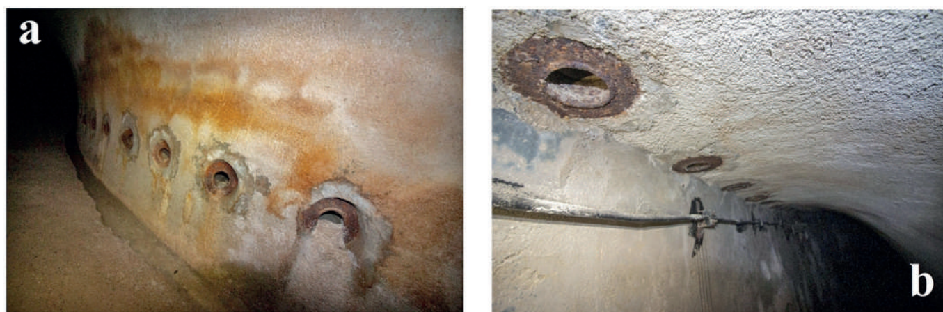
Fig. 6 – Pipes for water injection: a) horizontal injection; b) vertical injection (photo G. Monteleone).
