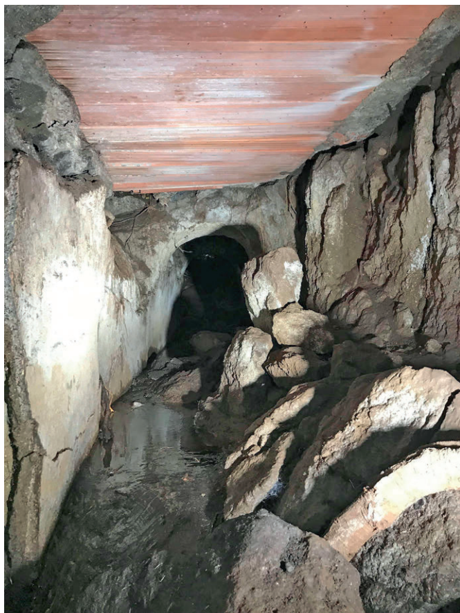
Fig. 5 – The collapsed part of corridor E with the refurbished ceiling (photo A. Schatzmann).
