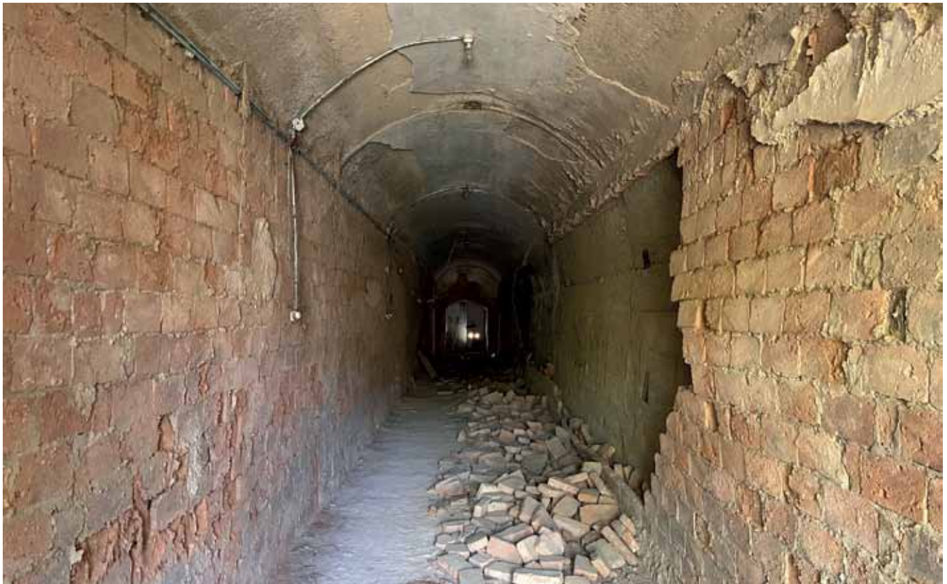
Fig. 5 – View of the tunnel from the entrance. In evidence, the masonry partition wall used for creating the air shaft, partially collapsed as shown in the right side of the photo (photo M. Cangemi).
