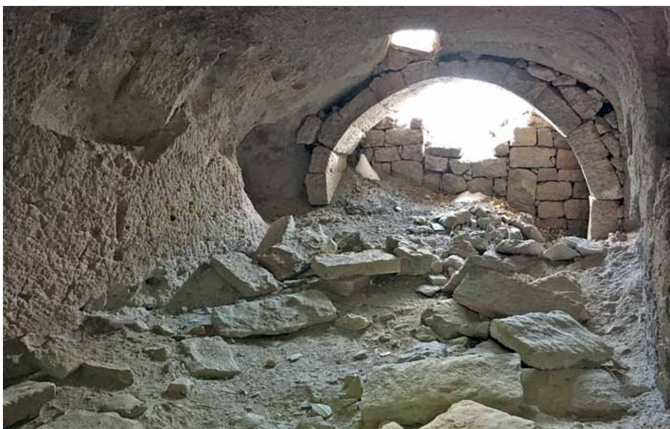
Fig. 13 – Chamber (F) of Derevank Monastery towards the north, with a stone arch at the entrance, closed by squared stones, partially collapsed (photo A. Yamaç).
